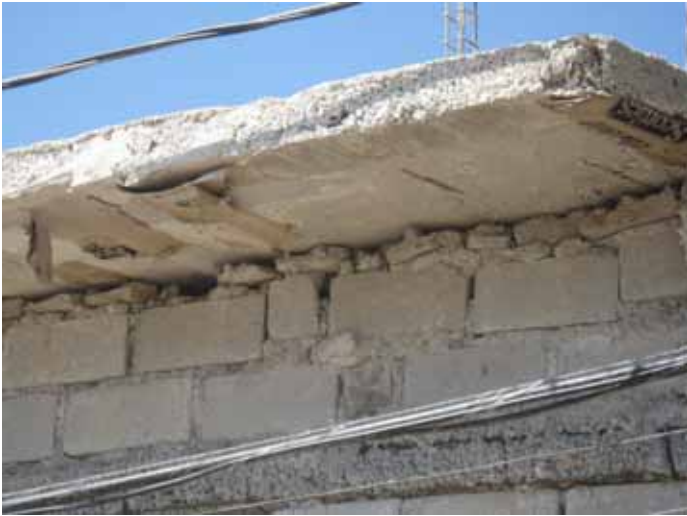
Figure 5 No Roof to Wall Connection
