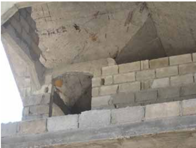
Figure 19 Lintel to Interior Wall (not connected to roof)
