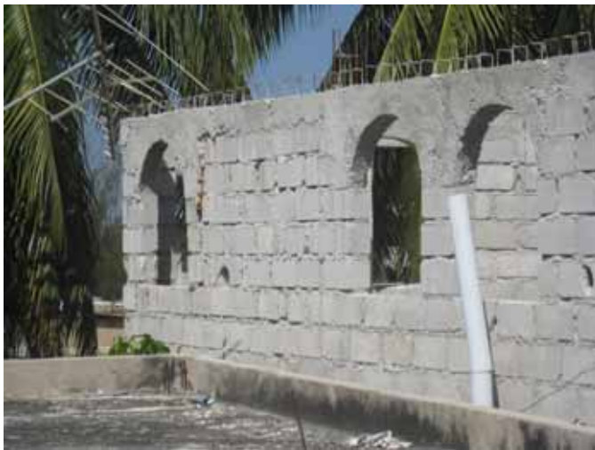
Figure 15 No Interior Wall Reinforcement (house under construction)
