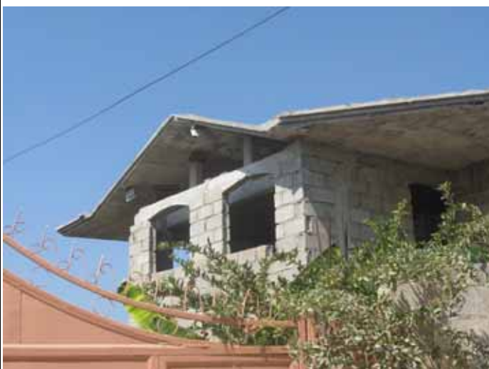
Figure 7 No Roof to Wall Connection (house under construction)
