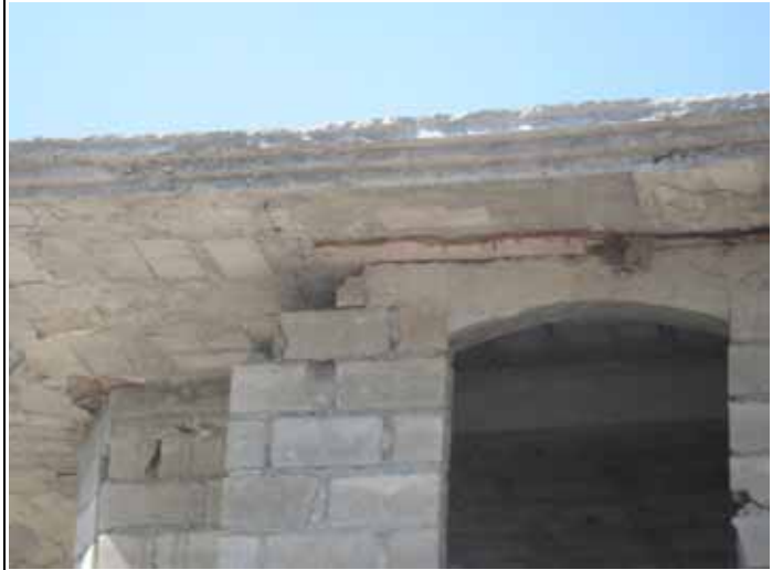
Figure 6 No Roof to Wall Connection
