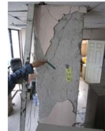
column shear cracking
