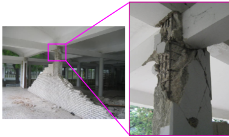
column shear failure
