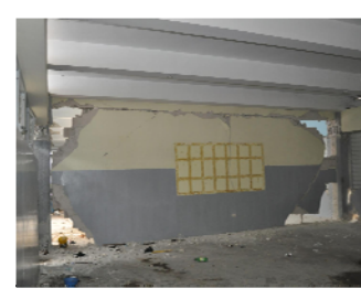
masonry wall failure
