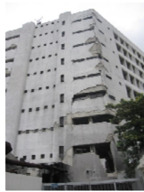
wall pier failure
