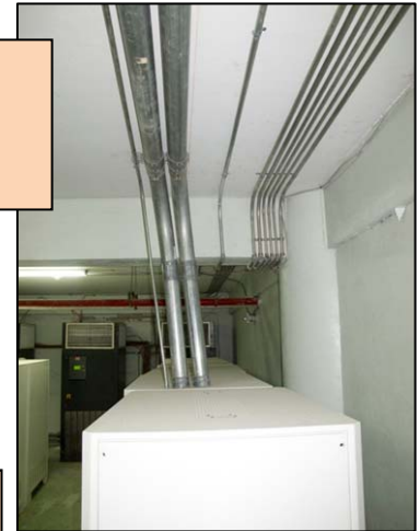
Unanchored UPS system (Digicel)
