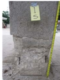
column base damage
