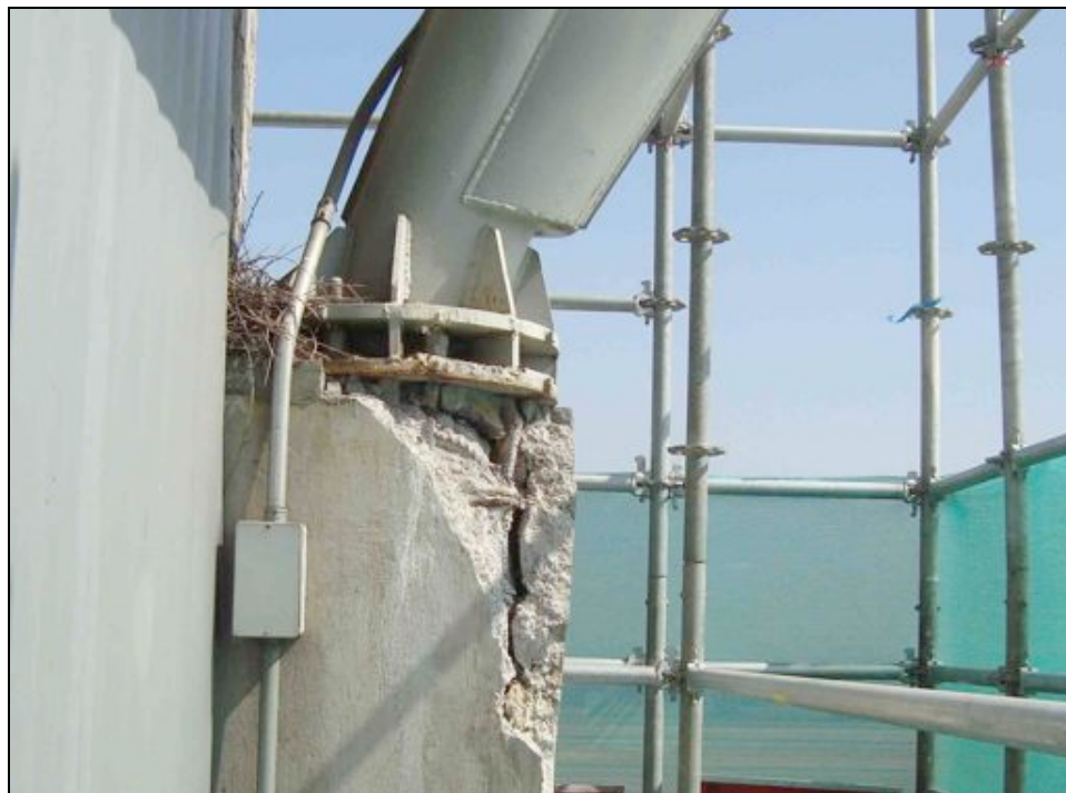
Santiago Airport control tower damage of the four anchor points of the cab structure
