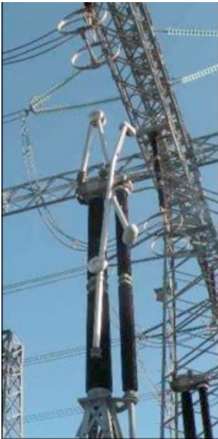
Pantograph disconnect switch
