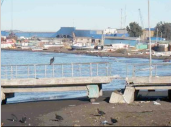
Concrete pier moved towards shore due to lateral spread lateral spread
