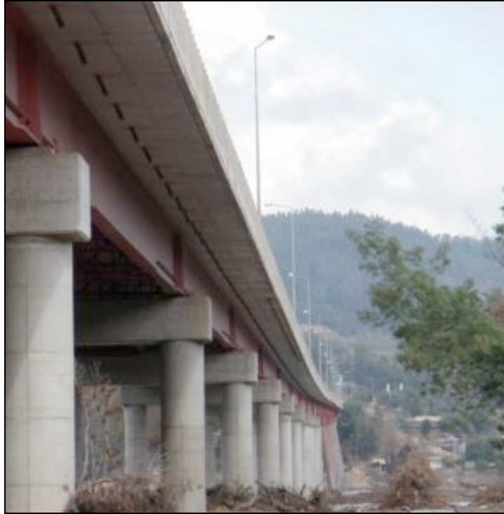
Tsunami damage to bridge in Constitución. The bridge girder was lifted by the tsunami and moved inland about 1 ft for a distance of about 6 bents. During the TCLEE team visit on April 16, 2010, the bridge traffic was being controlled to one lane of traffic. Team members witnessed official search activities for missing persons.
