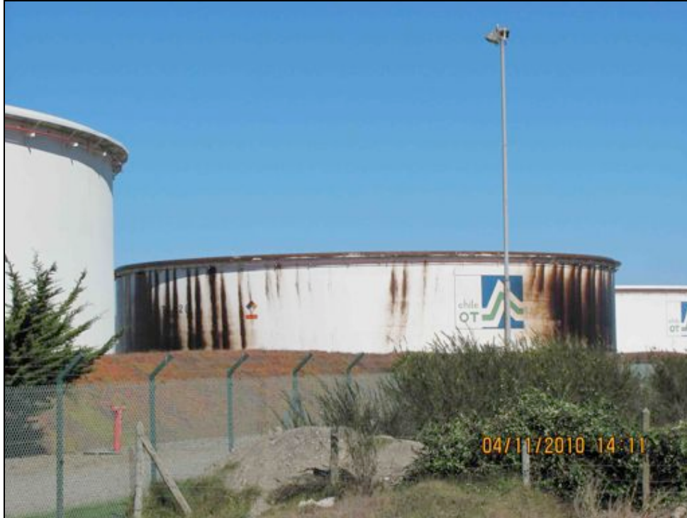
Oil tank sloshing spill over the rim
