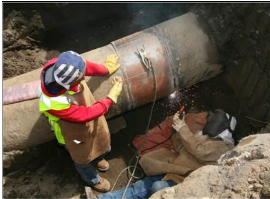
Damaged Large Diameter Welded Steel Water Pipe (Courtesy WWPP Chile)
