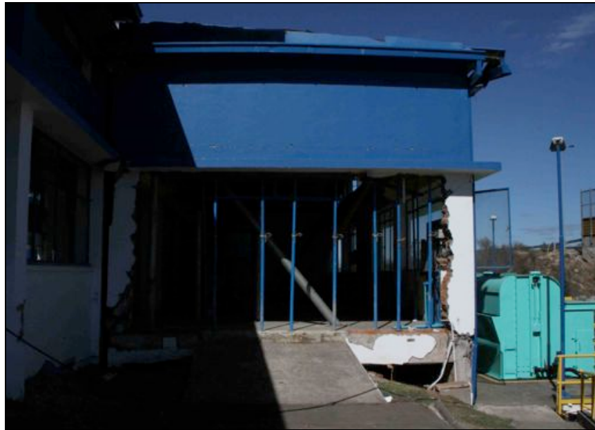
Collapsed wall at Concepcion Water Treatment Plant Raw Water Pump Station
