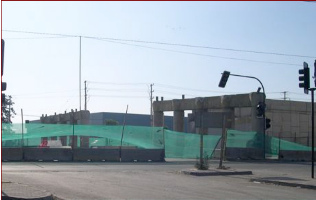
One of the overpasses damaged, this is the highway towards Santiago Airport.
