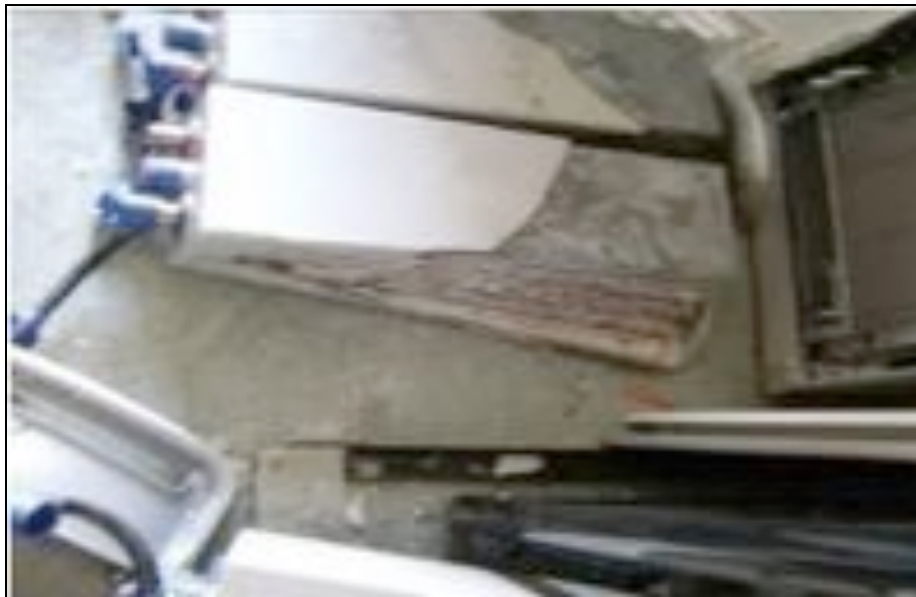
Unsecured batteries on unanchored battery rack fell off the rack and damaged (Courtesy Carlos Urzua Acuña)
