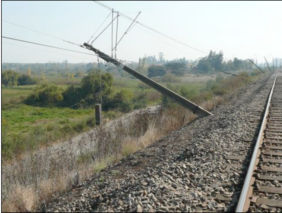
Overhead power line for electric power rail cars failed
