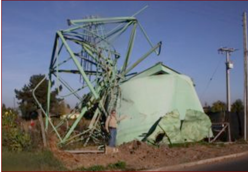
Typical Collapsed Elevated Small Steel Tank (Constructed 1999)
