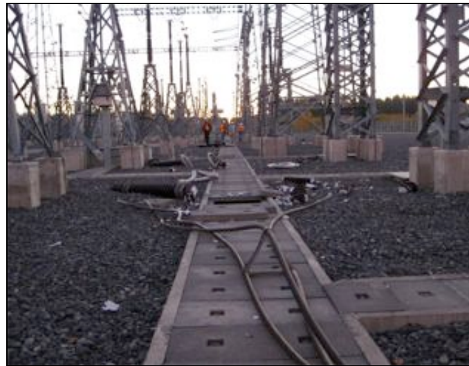
Damaged candlestick style live-tank circuit breakers
