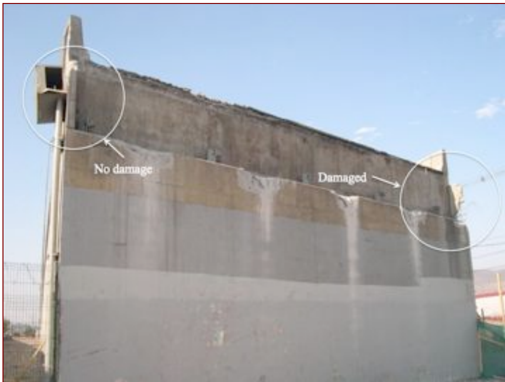
Note the circled areas, showing rotation of the deck.
