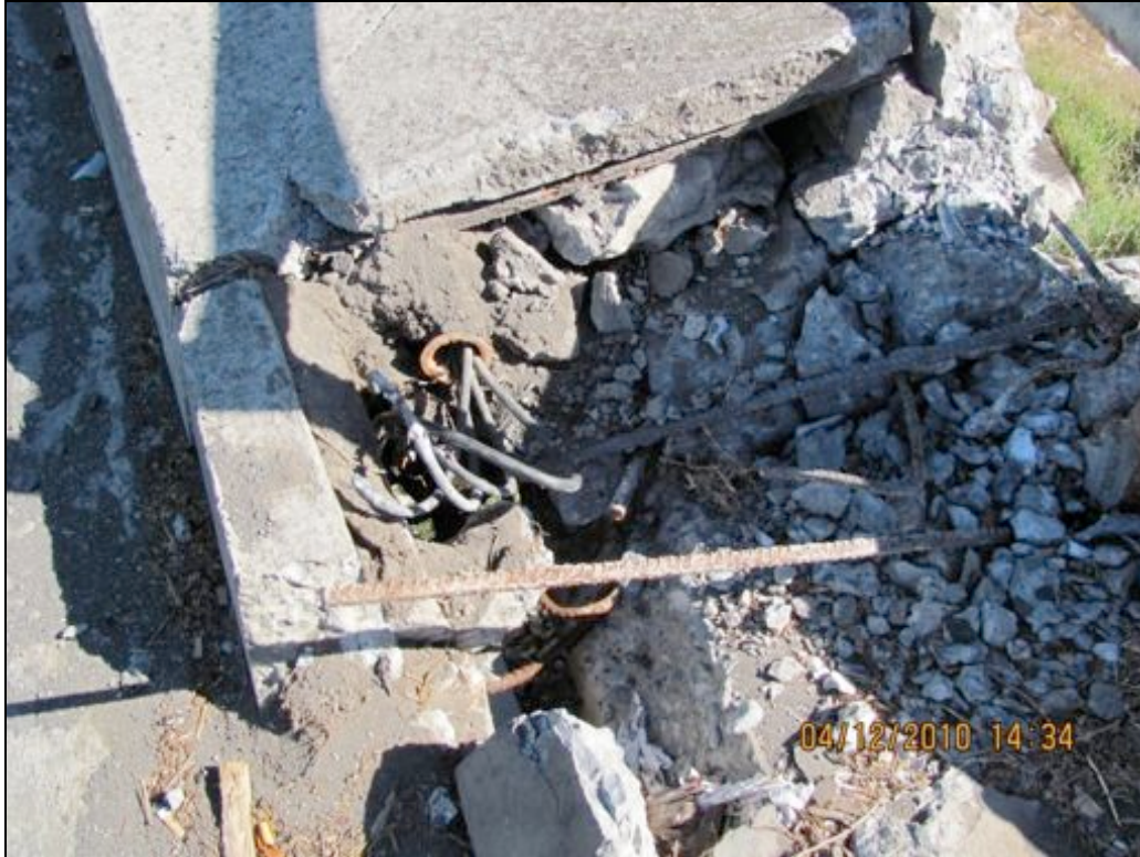
Co-located power and telecommunication cables along the damaged Juan Pablo II bridge over the Biobío River in Concepcion.
