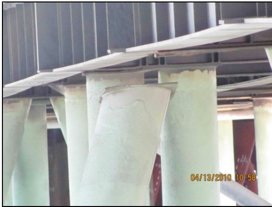
Pier 1: a few pile supports with broken weld were observed
