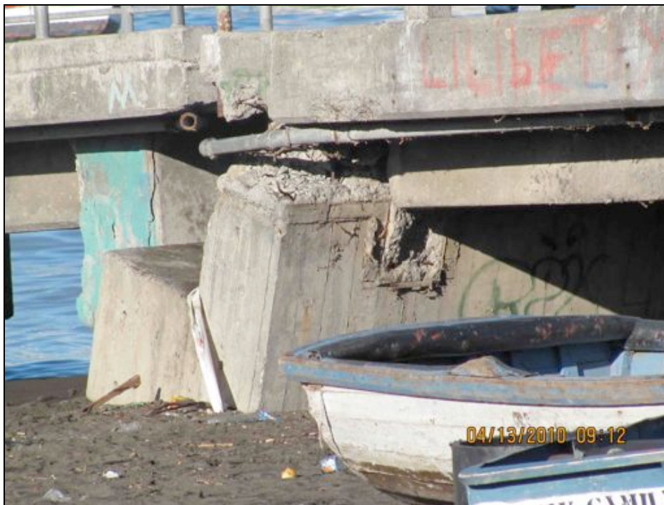
Liquefaction and lateral spreading damage at Coronel fishing port. Note the damaged lifeline.
