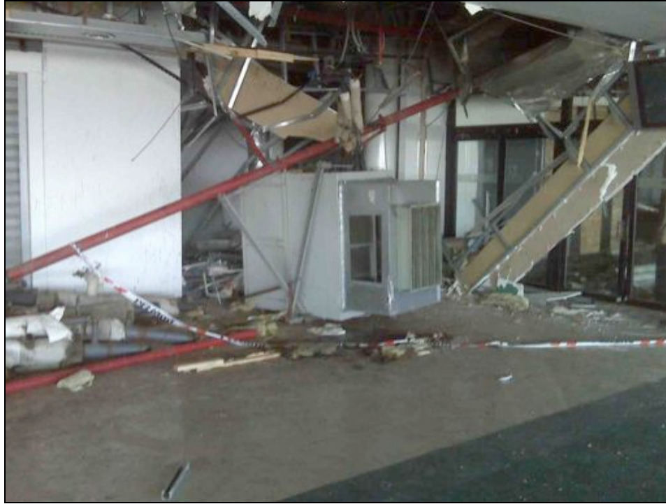
Non-structural damage of Santiago Airport passenger terminal on the departure level (courtesy of Juan Pablo Muñoz)
