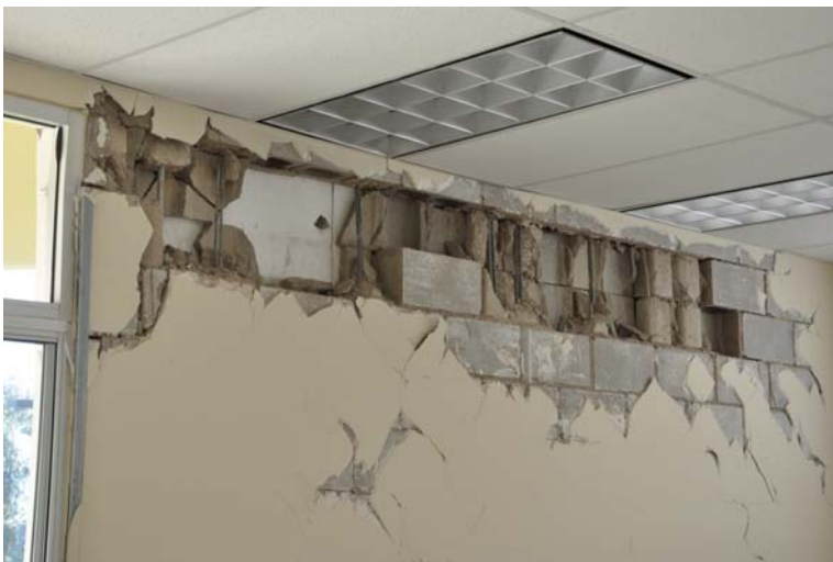
Figure 9. Damage at the UABC (Universidad Autonoma de Baja California ( N32.6320°, W115.4444°): (top) typical exterior damage of low-rise masonry construction, (middle) interior ceiling damage, and (bottom) damage to partially grouted CMU walls.
