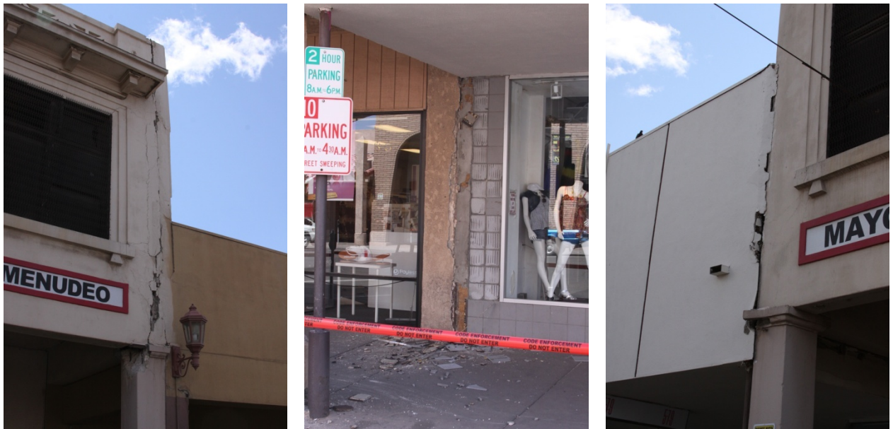
Figure 6. Damage due to impact of neighboring structure storefronts in downtown Calexico (images courtesy of professional photographer Joseph Llausas - taken April 5, 2010).
