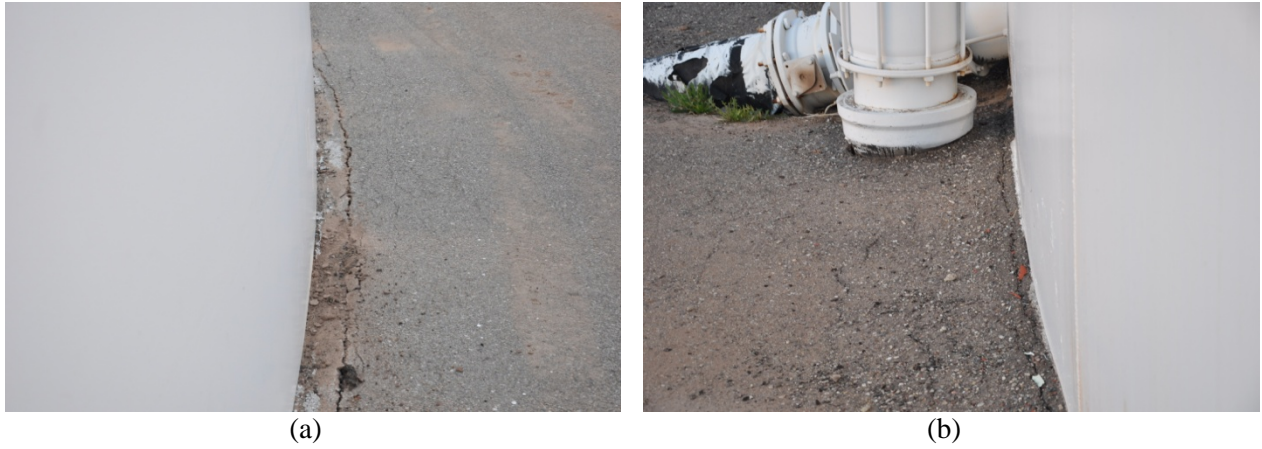
Figure 5. Evidence of dynamic foundation movement (a. N32.6703°, W115.5049°; b. N32.6704°, W115.5048°). (note cracks in pavement and separation between pipe and pavement). Calexico Water Treatment Plant.
