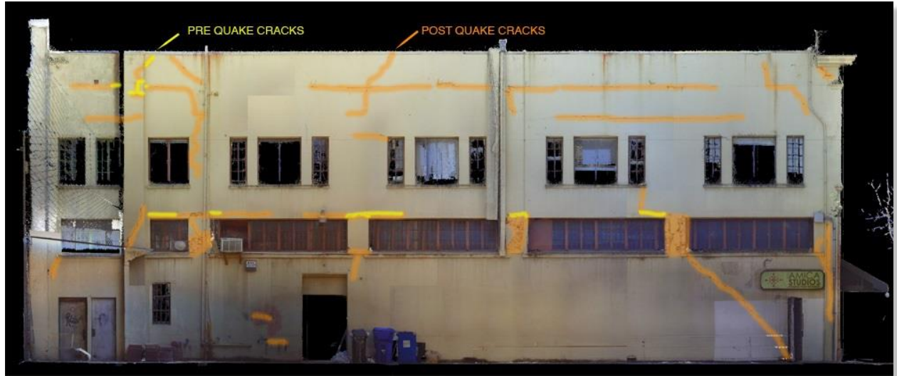
Figure 6 – Post-quake West wall showing pre- (yellow) and post-quake (orange) cracking
