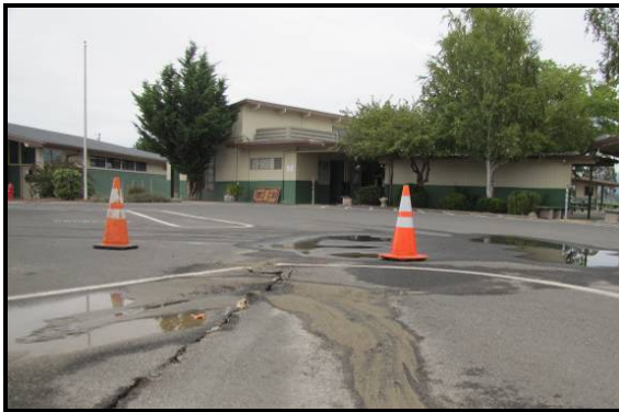
Ground rupture in an elementary school parking lot south of Napa resulted in fracture of underground water piping.
