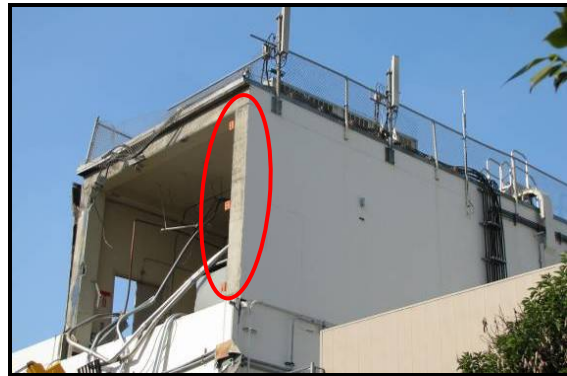
Precast concrete wall panel connections failure at a local telecom hub damaged HVAC system at this critical facility.
